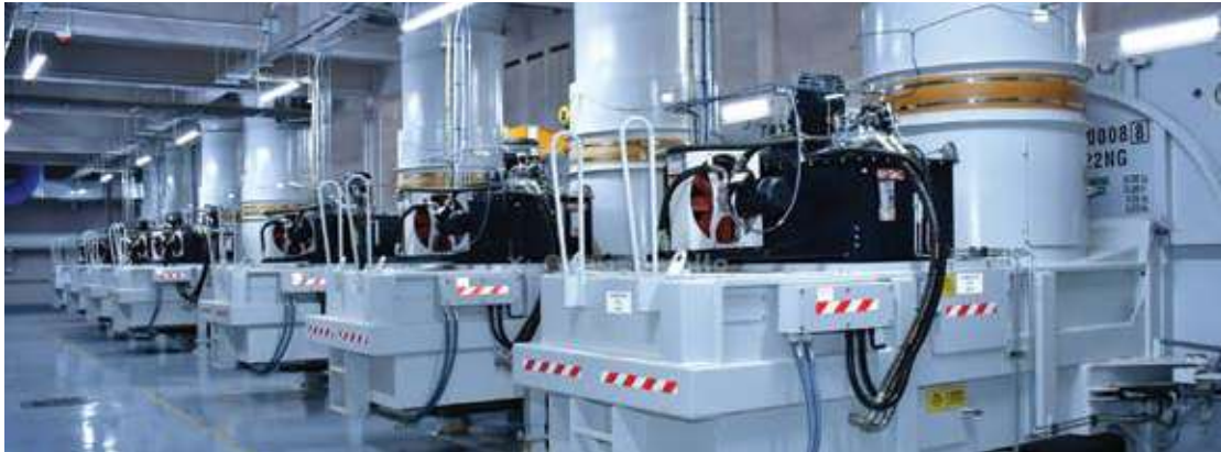
The continent's first automated pneumatic solid waste management located at the Konza Technopolis.
